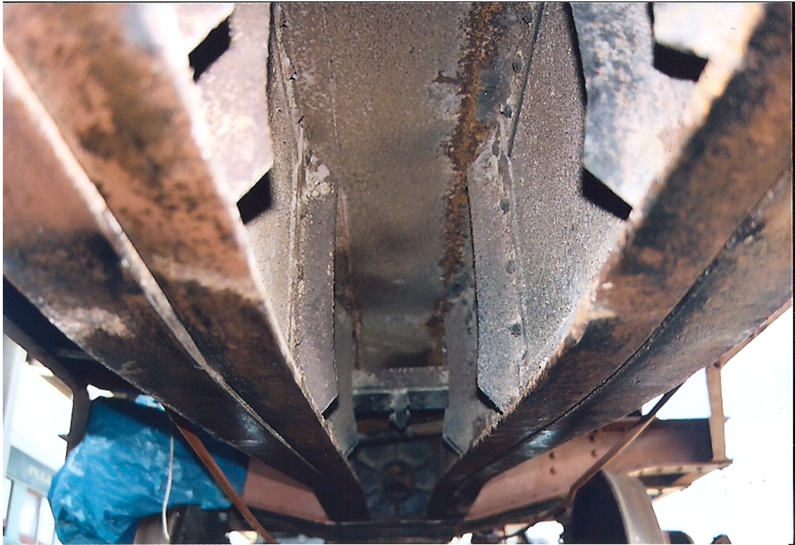
Figure 10. B end center sill before cleaning
