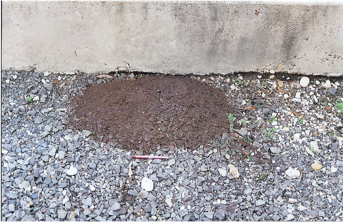
Figure 15. Rust removed from the B end bolster. The 6-inch pen is for scale.
