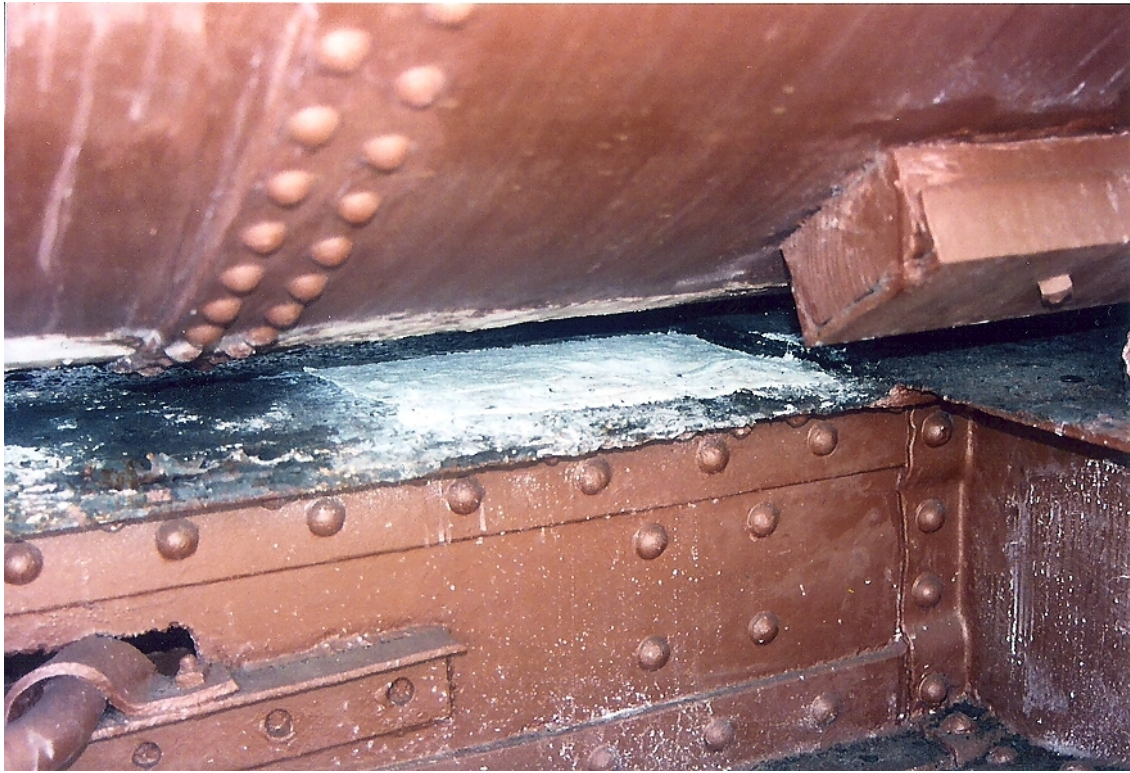
Figure 14. Rusted hole in the center sill plate patched with plaster cloth
